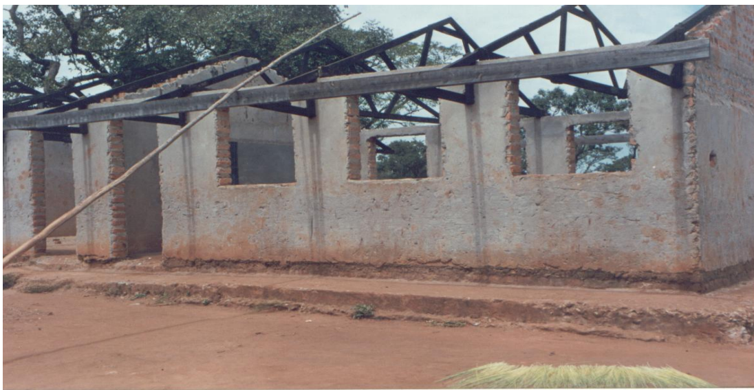
Opiu Primary School. The roof was blown off. Now the pupils study from under a mango tree.
